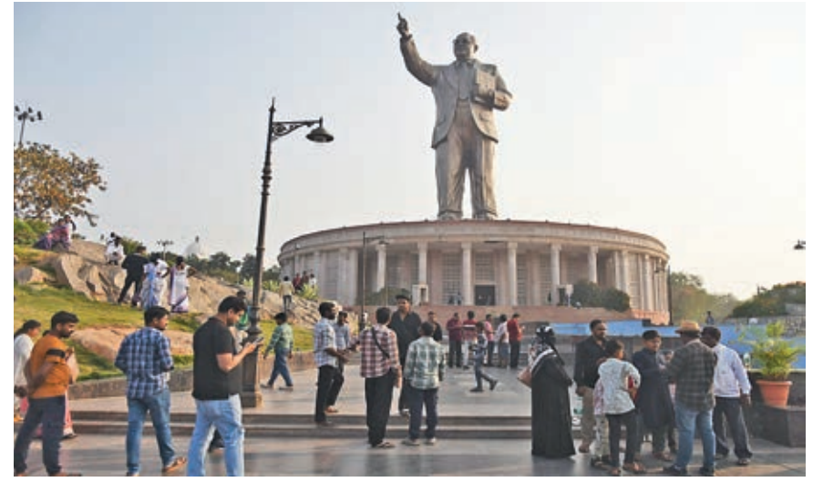
Visitors can now see the Ambedkar statue near NTR Marg from afar as the entrance ceiling is still damaged, fountain nonfunctional, and museum remains closed.
